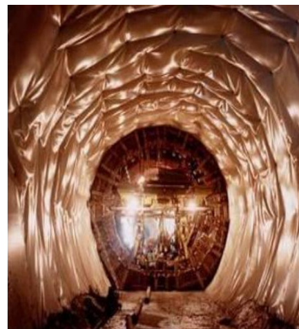
Figure 9. Geomembranes in Tunnel [3]
