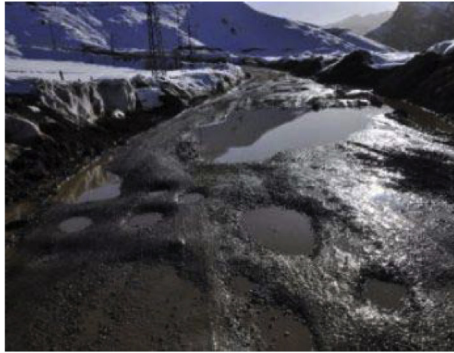
b) Cuts in road due to water (Beyaz Gazete, 2013)
